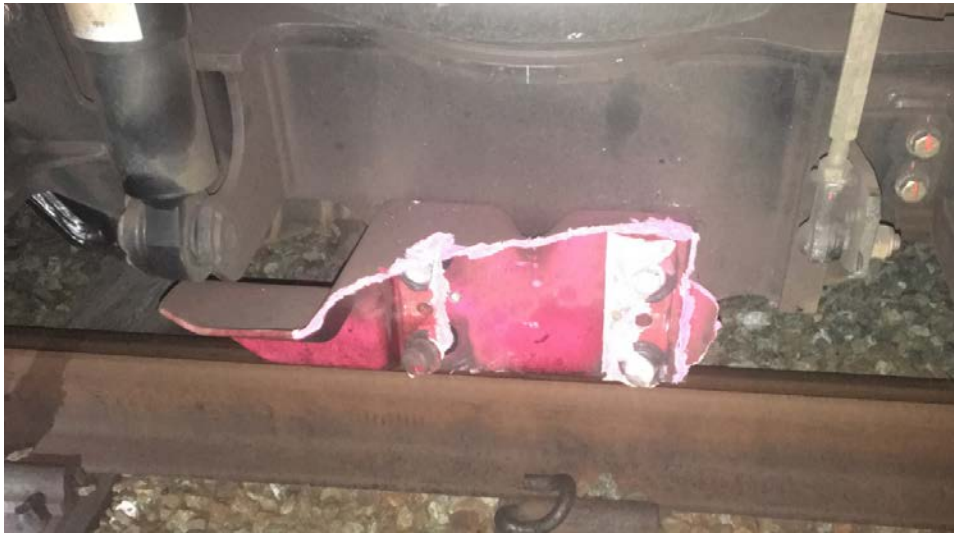
Photo 3 – Damaged Collector Shoe Assembly
