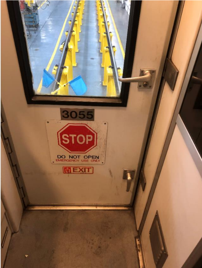
Photo 5 – Bulkhead door was rubbing against the threshold plate
