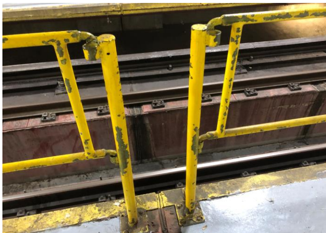
Photo 2 –Some open pits railings have unprotected openings
