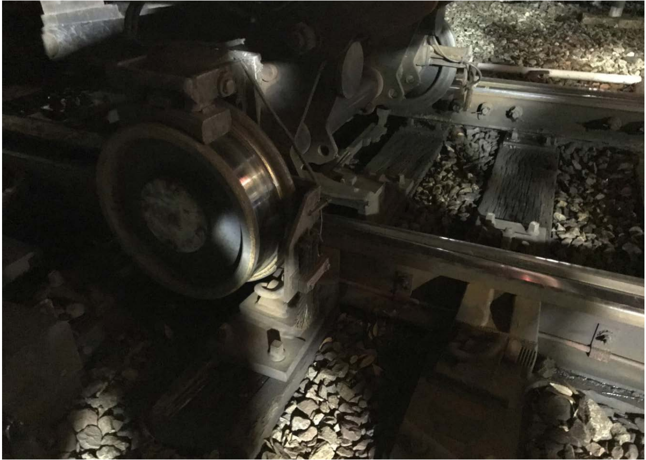
Photo 4 - Final Resting Point (FRP) 3-6 inches away from derailment location.
