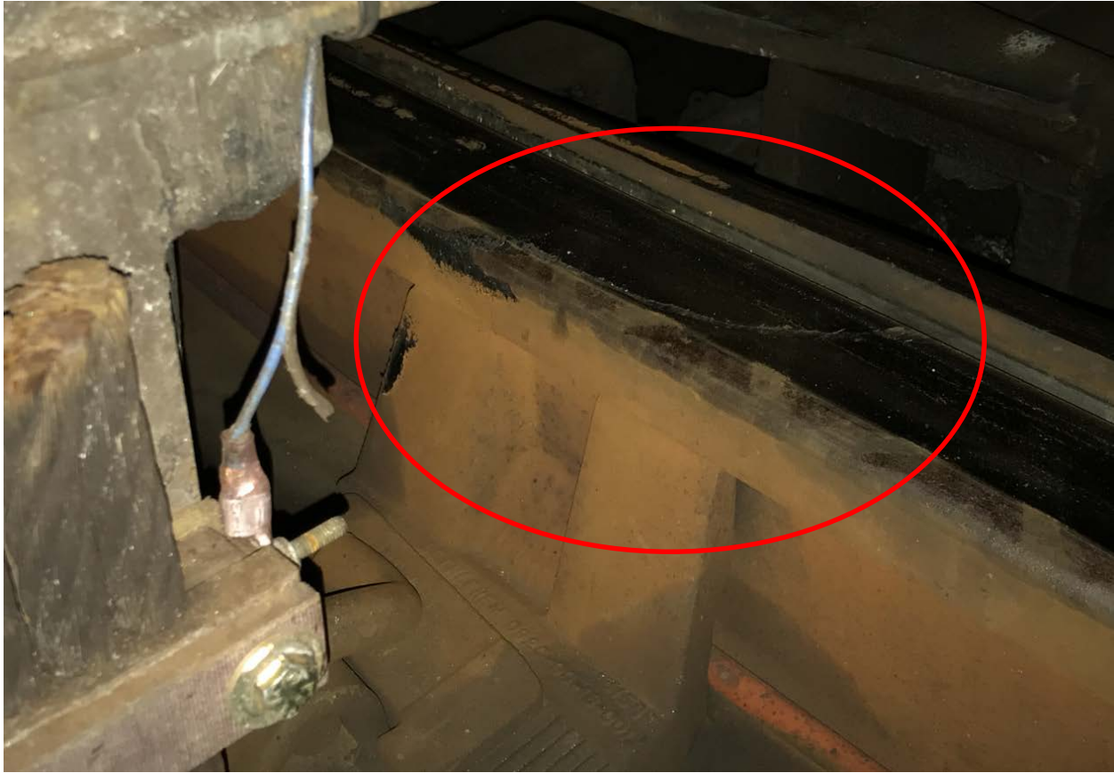
Photo 3 – POD markings on the head of the left side running rail with flange grease markings within the switch point.
