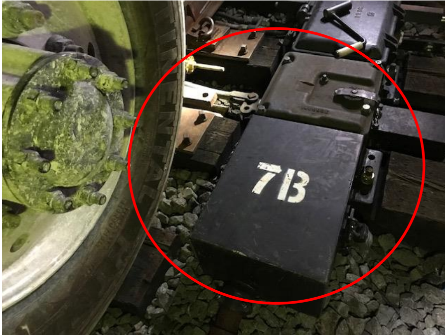
Photo 1 – 7B Switch indicates clamped switch points.
