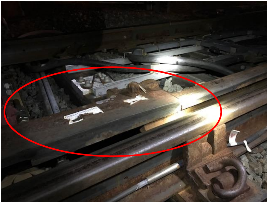
Photo 2 – The rider rear side HRU wheel climbed the housetop of the switch and derailed.
