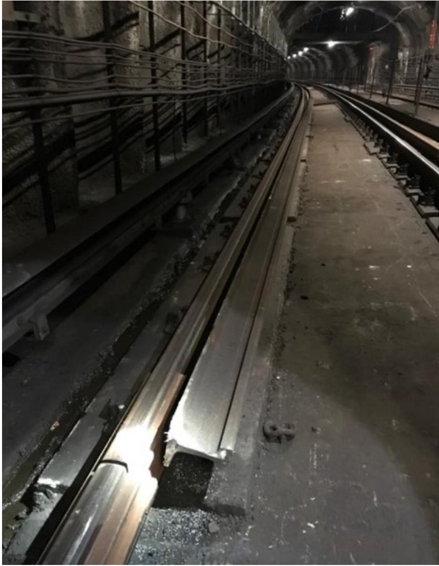
Photo 3 – Old stringer rail positioned on top of the clips and fasteners on arrival in the proximity of CM A2-084+00 (Ten) 10-feet away from SM04.
