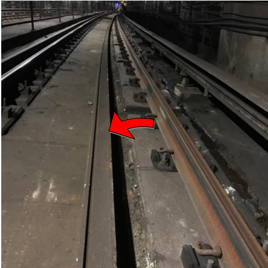
Photo 1 – Old running rail fall direction (Rail distance from the clips and fasteners varied at both ends of the work area).
