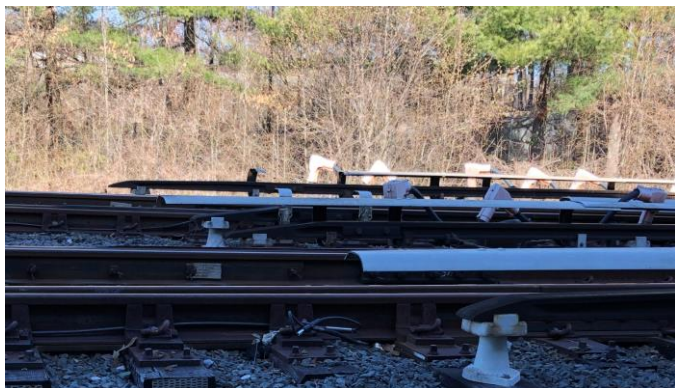
Photo 3 – Some third rail covers were missing
