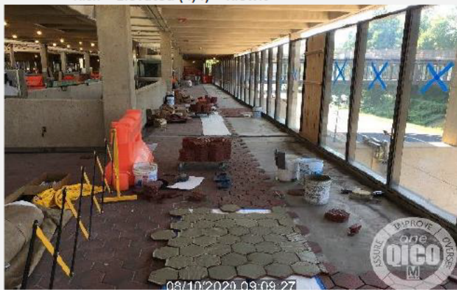
9. Missing tile and handrail along the wall (Work in progress) Mezzanine, south side Risk – Elevated (4,4) – Kiewit
