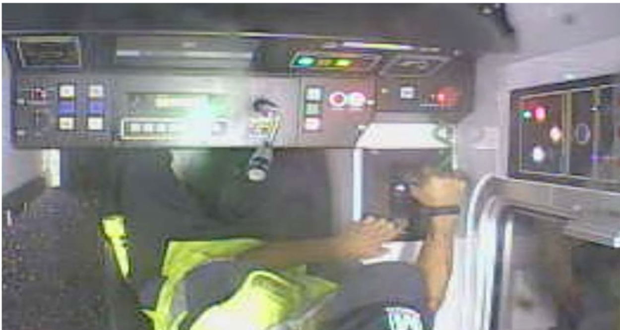
Photo 5: After that, the CMNT Technician went back in the lead car, keyed up, continued DI check, then depressed the overtravel button and moved the MC to the coast position three times, subsequently achieving a brakes off indication on the console.
