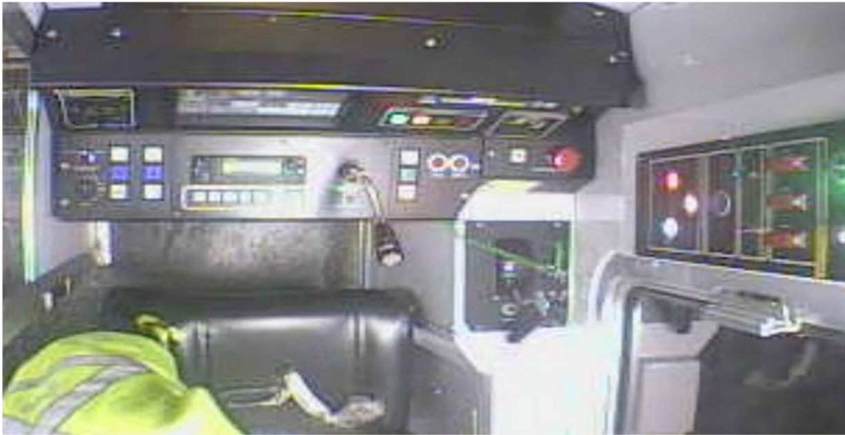
Photo 4: The CMNT Technician is observed shortly after keyed up in car 7668 installing seals on the K and L panel behind the Train Operator seat.
