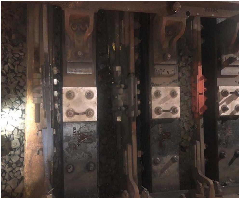
Photo 4 – There were no anomalies found to switch 7A/B.
