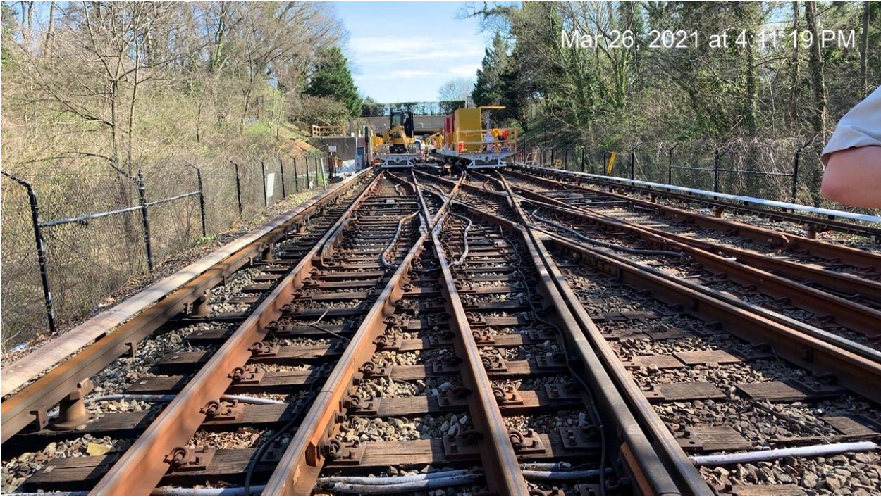
Photo 4: Switch located near Arlington Cemetery Station.
