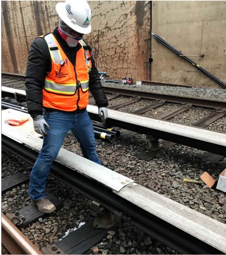
Figure 3 – The Injured Contractor assumed a braced position with firm footing, straddling the third rail.
