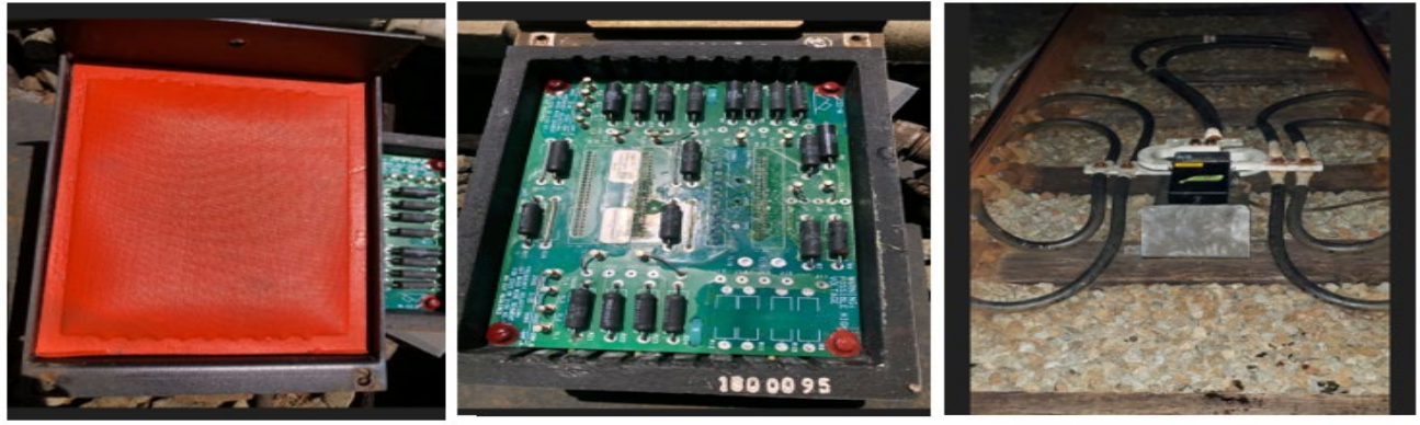
Image 1 - Photo #1, the cover of the Wee-Z Bond with the anti-vibration pad saturated in water. Photo #2, corrosion on the control board. Photo #3, replacement Wee-Z Bond installed.
