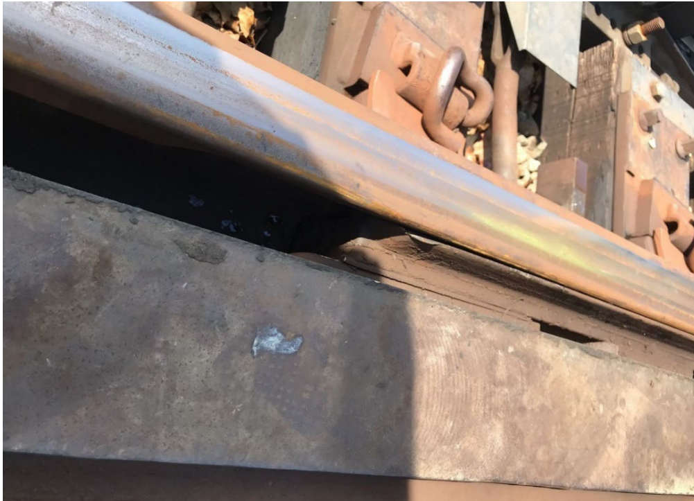
Photograph 3 – Switch 17A was not tucked during the red signal overrun and sustained a slight bend at the tip of the point.
