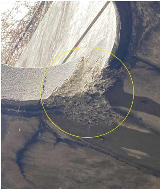
Image 7 - Superficial chipping of the portal was observed during an inspection by TRST.
