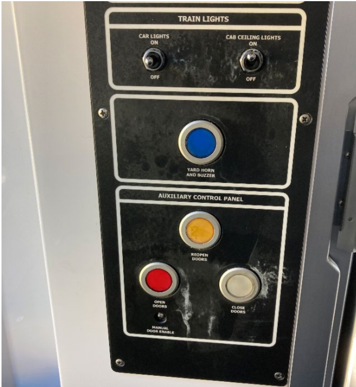
Train operator door control panel
