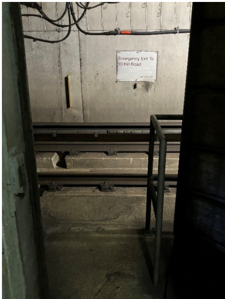
Figure 3: This image shows the proximity of the emergency egress door to the roadway.
