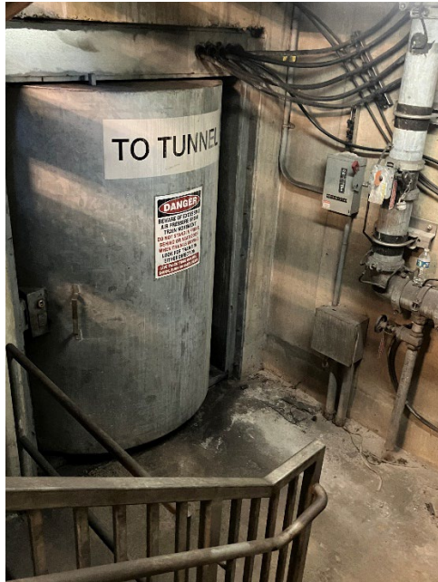
Figure 1: This shows the emergency egress door that was used to access the roadway.
