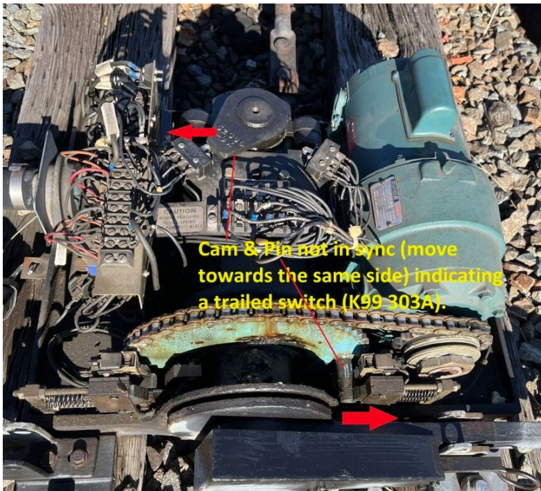
Image 4 – Image of Switch 303A, indicating a trailed switch.
