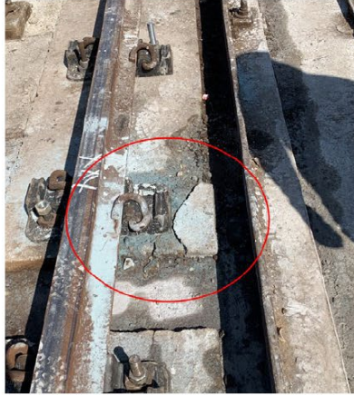
Figure 13: Damaged Grout Pad
