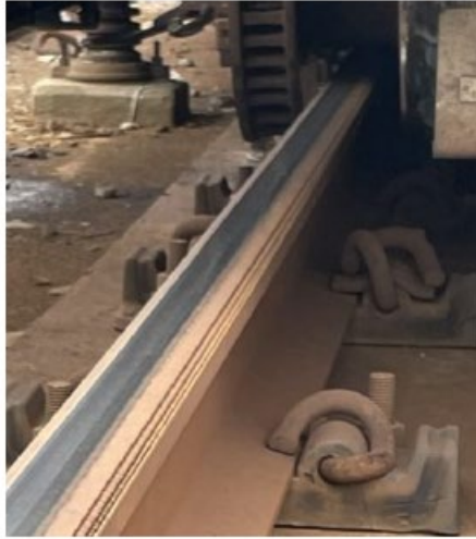
Figure 7: Derailed Right Wheel of Lead Axle
