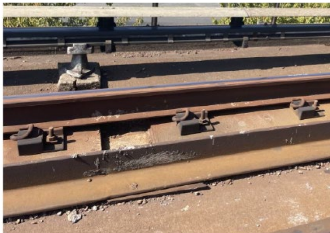
Figure 12: Damaged Insulator Grout Pad
