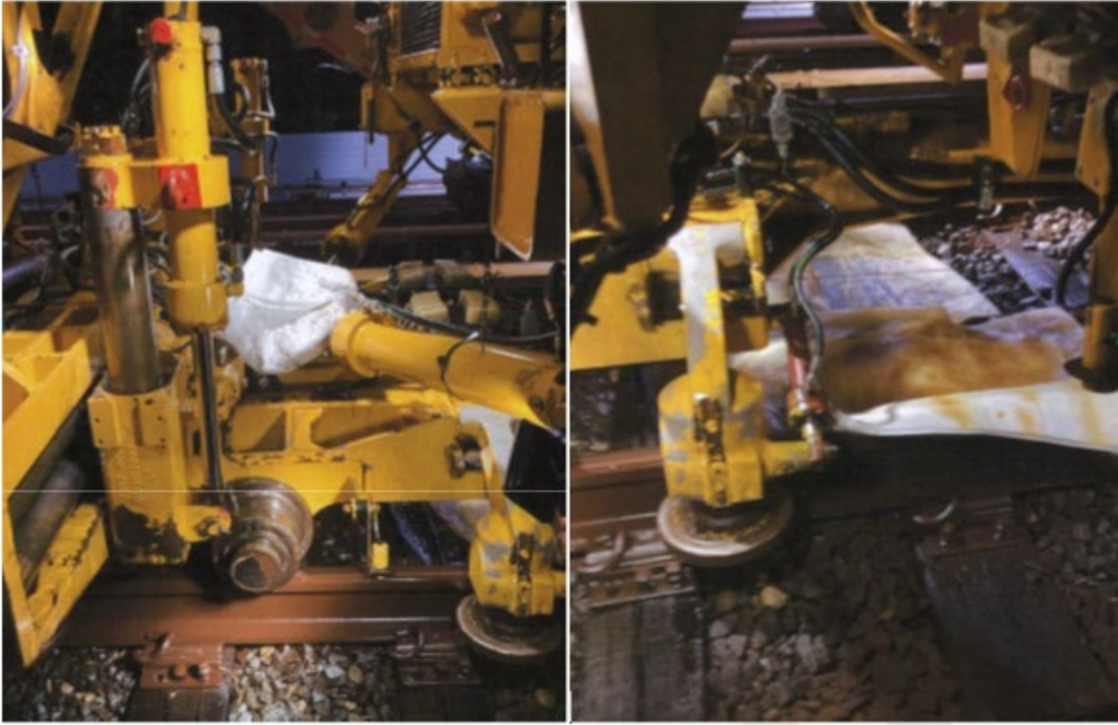
Figure 2 - Tamping Unit T004 leaking hydraulic fluid onto Absorbent pads.
