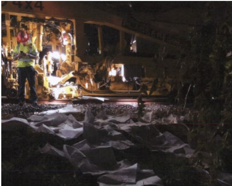
Figure 10 - depicts absorbent pads leading down the embankment from Tamping Unit T004 containing the hydraulic fluid.
