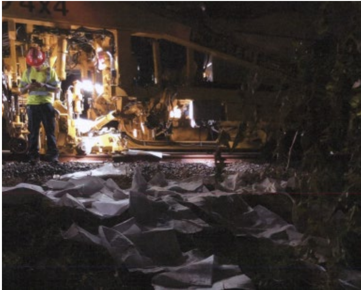
Figure 3 - depicts absorbent pads leading down the embankment from Tamping Unit T004 containing the hydraulic fluid.
