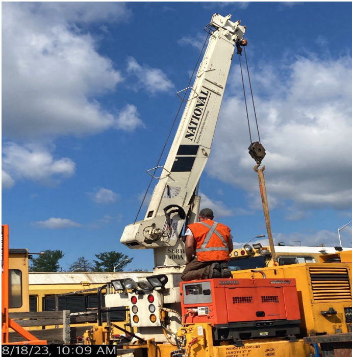
Figure 11 – Inspection of the winch brake on the boom of PM-578.
