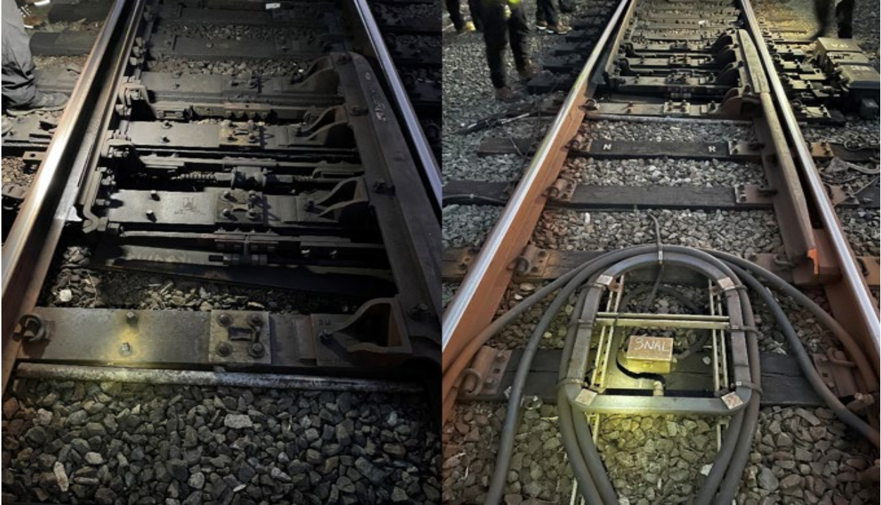
Figure 5 - depicts switch 3A with no damage to the switch or switch point.
