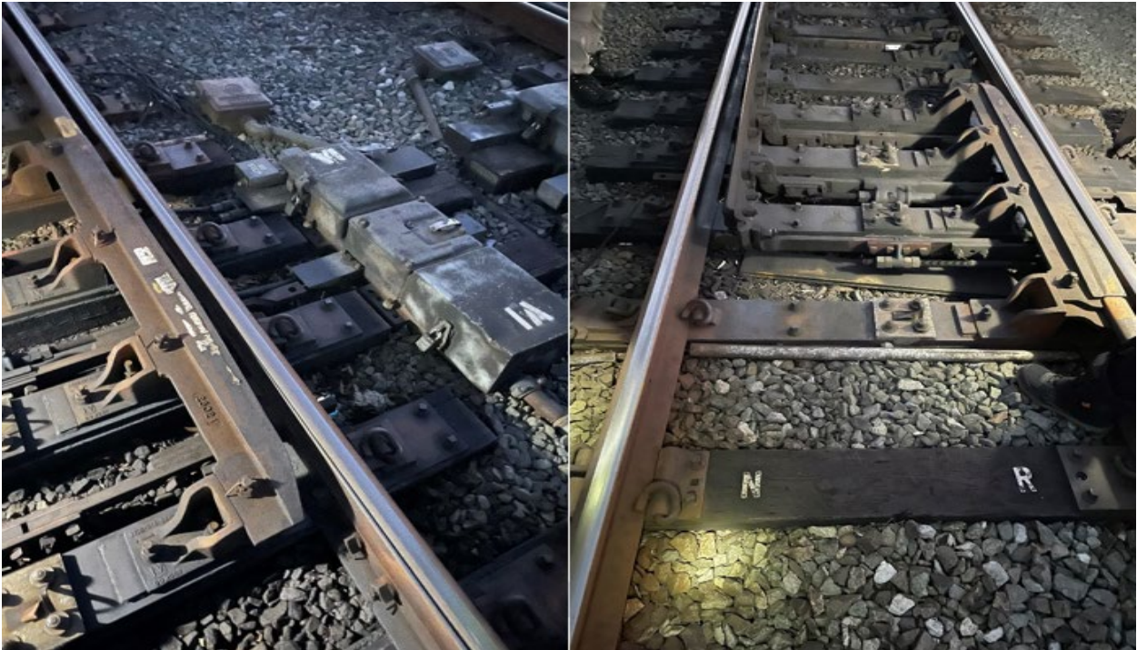
Figure 6 - depicts switch 1A with no damage to the switch or switch point.
