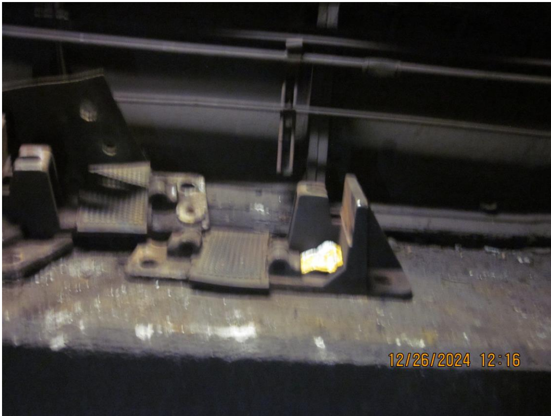
Obstructions (Removed track materials)
