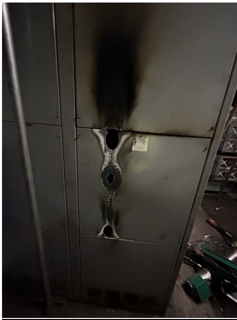
Image 1 – UPS Gear after the explosion.
