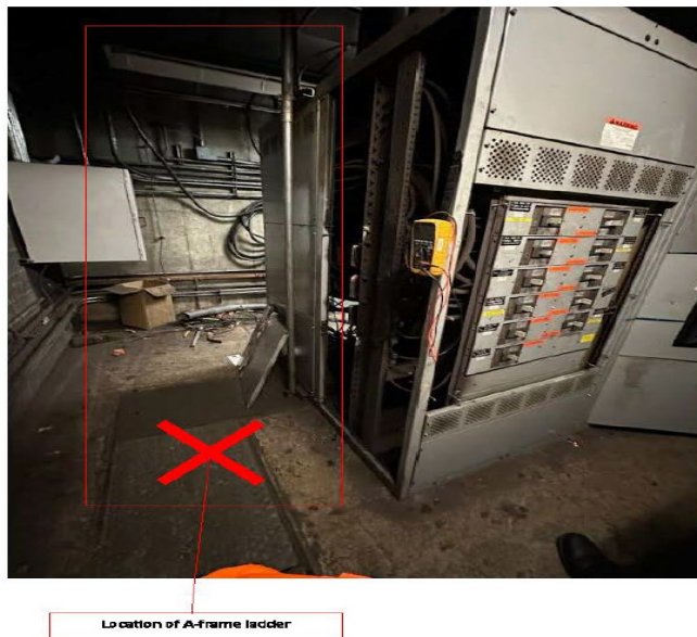
Image 5 - AC Switch Room Side B
