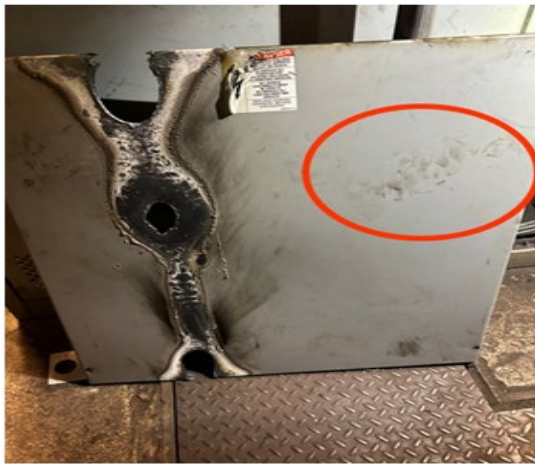
Image 3 – Footprint on the UPS Gear Panel Cover discovered after being removed.
