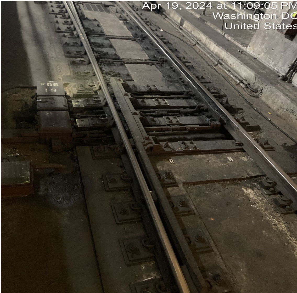
Figure 5- Switch 1B in normal position. (no damage)
