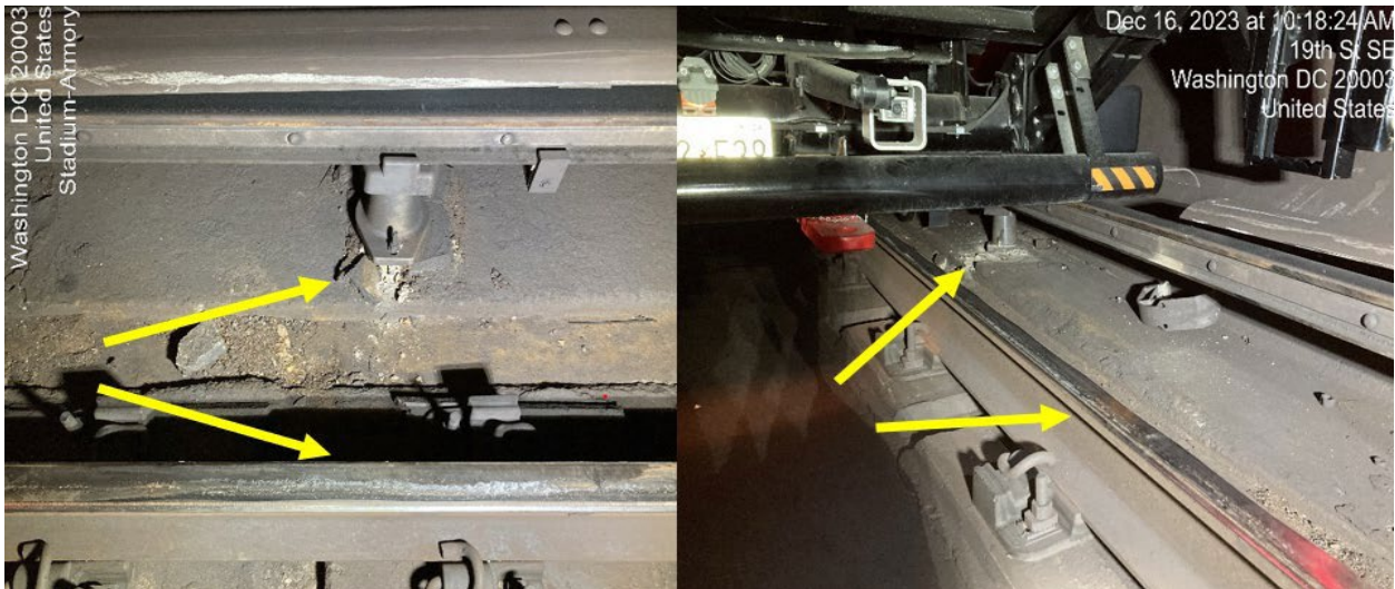
Image 3 & 4 – Images depict damage to running rails and insulators.
