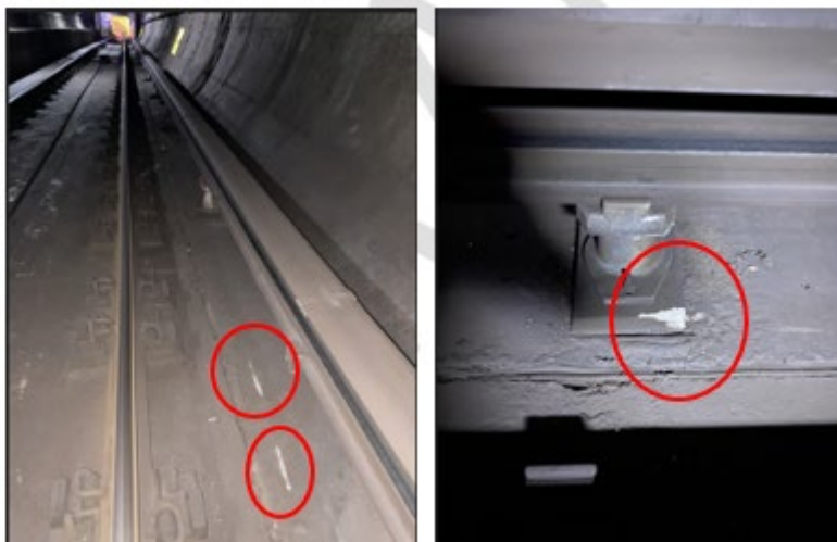
Image 17 – Image of the scuffs along the invert and third rail grout pad.
