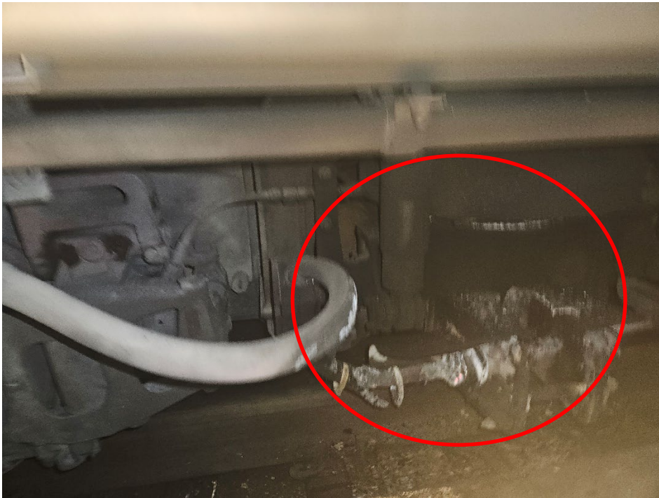
Image 12 - The above photo depicts a different angle of damage assessment of the #2 collector shoe assembly and power cable positioned on the front truck of Car 7663.
