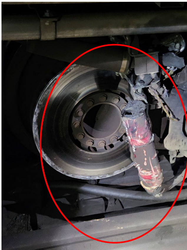
Image 13 - The above photo shows the collector shoe fuse dislodged from the missing collector shoe assembly and damage to the #6 brake disc on car 7663.
