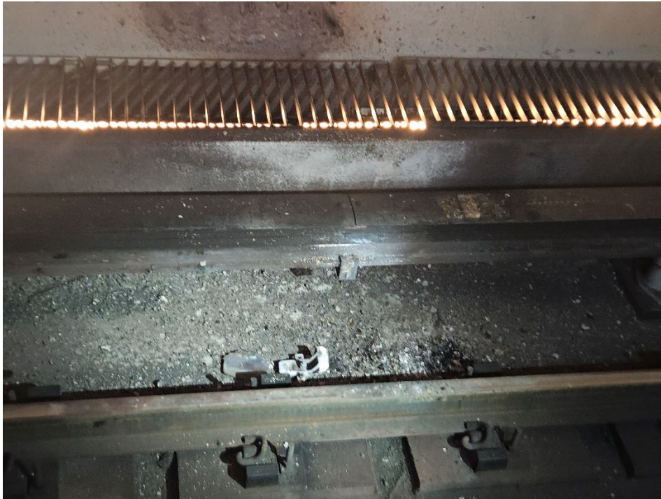
Image 10 - The above photo shows the arcing location at Eastern Market Station, approximately 450 feet from the 8-car marker.
