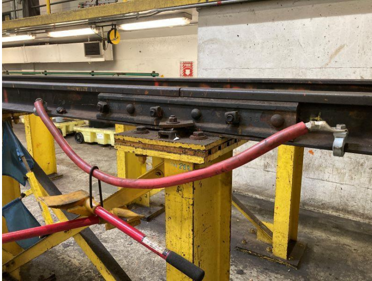
Photo 5: Negative return cable with temporary clamps being used to support a chock and presenting slack in the cable.
