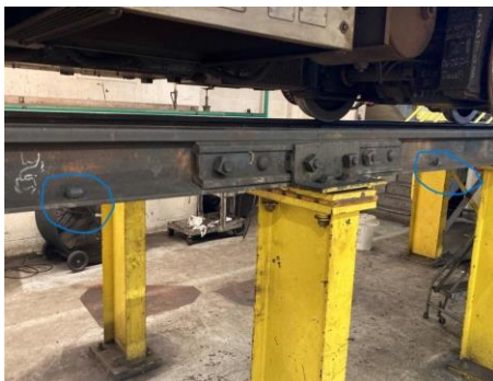
Photo 1: Track 2N showing missing negative return cable.
