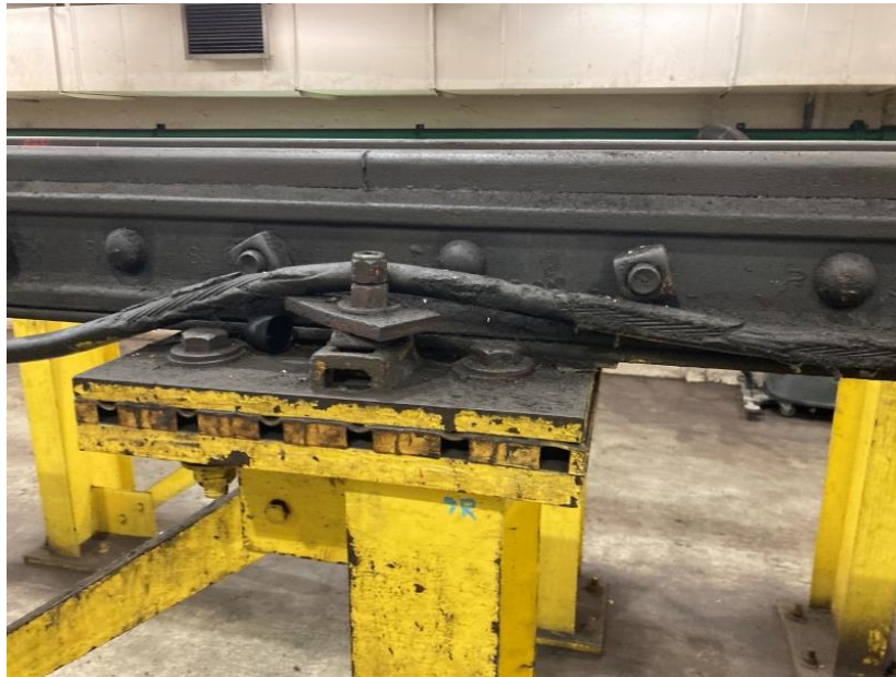
Photo 2: Negative return cable with insulated cover showing deterioration.
