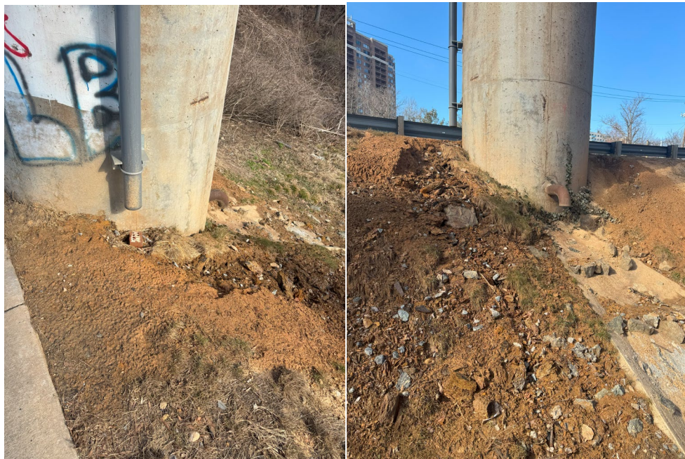
Photo 8 (left) soil erosion at pier A-5435. Photo 9 (right) soil erosion from a different angle at pier A-5435.
