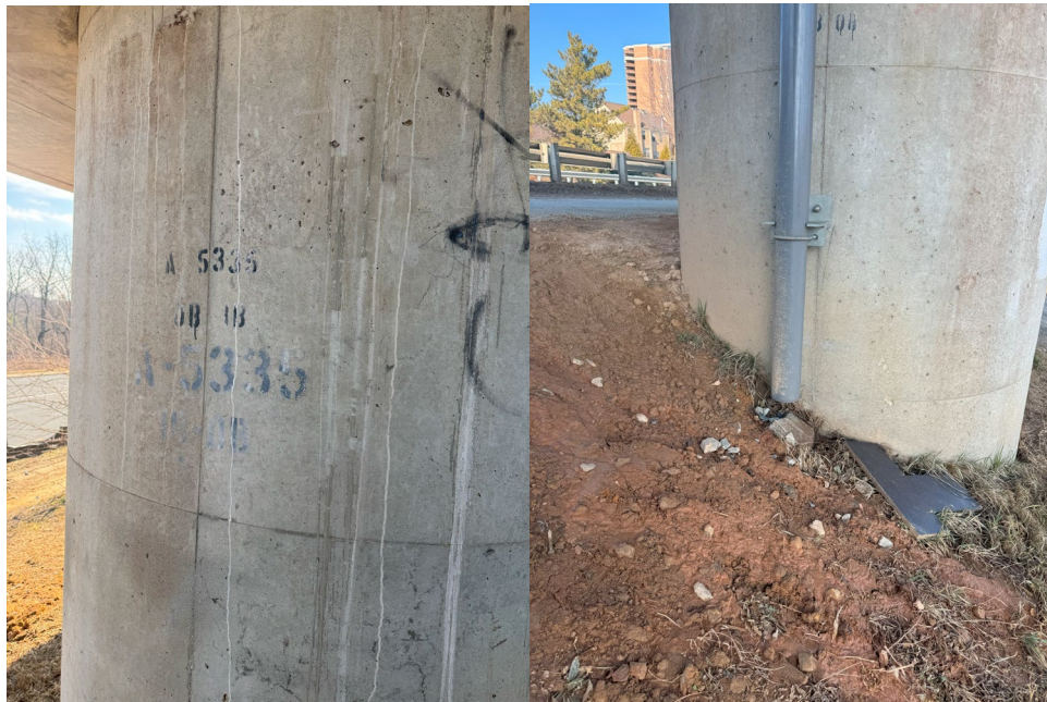
Photo 1 (left) faded pier identification at pier A-5335. Photo 2 (right) signs of erosion near downspout at pier A-5335.
