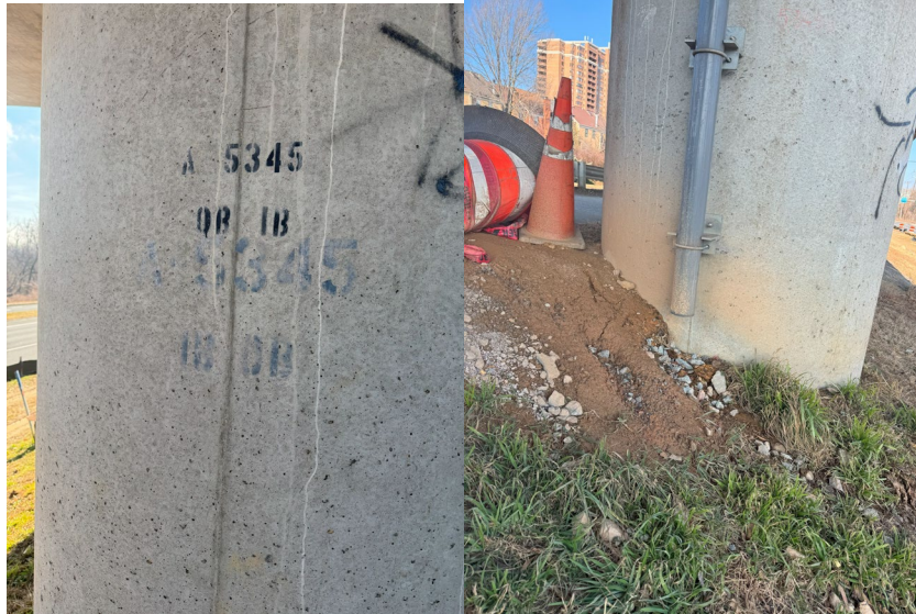
Photo 5 (left) faded pier identification. Photo 6 (right) exposed soil near base.
