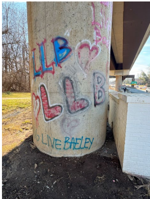
Photo 11 shows an unidentifiable pier north of A-5435.
