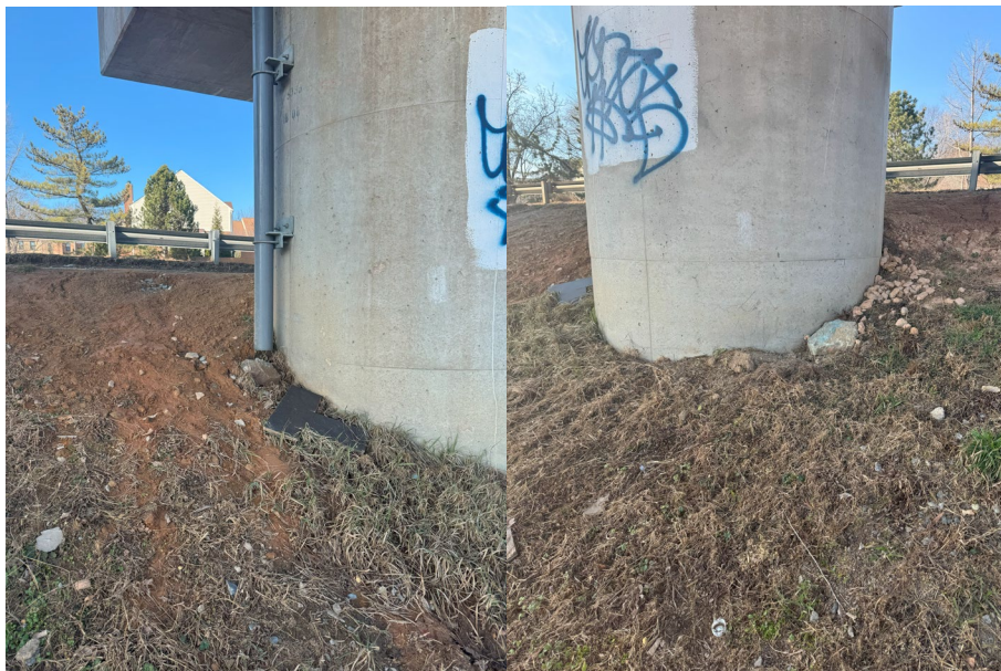
Photo 3 (left) Signs of erosion and exposed soil near base of pier A-5335. Photo 4 (right) opposite side of the same pier (A-5335).
