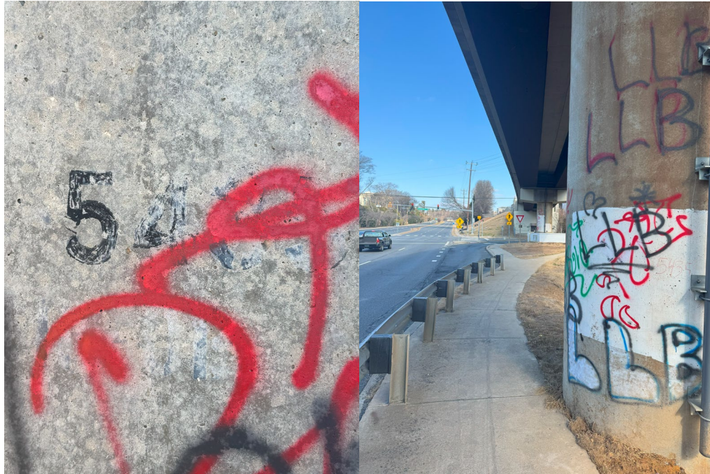
Photo 7 (left) graffiti and faded pier identification at pier A-5435. Photo 8 (right) pier A-5435 from sidewalk.
