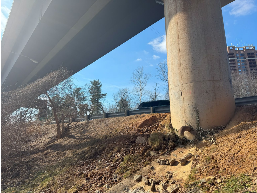
Photo 10 wider angle of pier A-5435 erosion on grade side.
