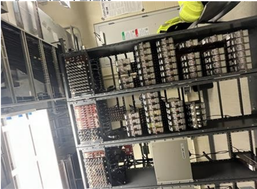
TCR Racks lp Relays rp .jpg
