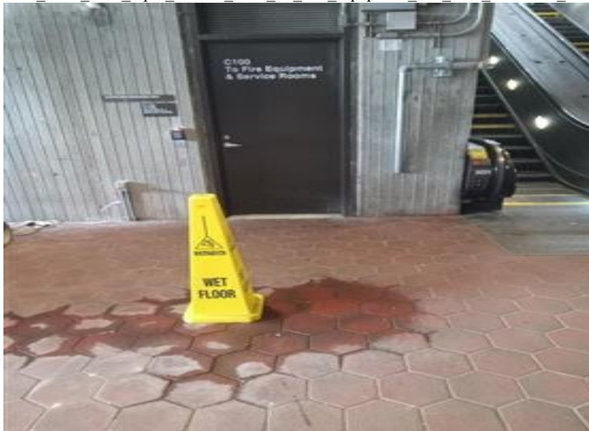
Leak From Roof Pipes Outside Door To Fire Equipment RM New Carrollton Station 032024.jpg
