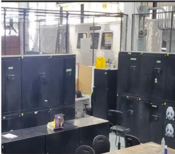
Outdated MSRPH in employee break-locker area at C99 Yard Alexandria Va.
