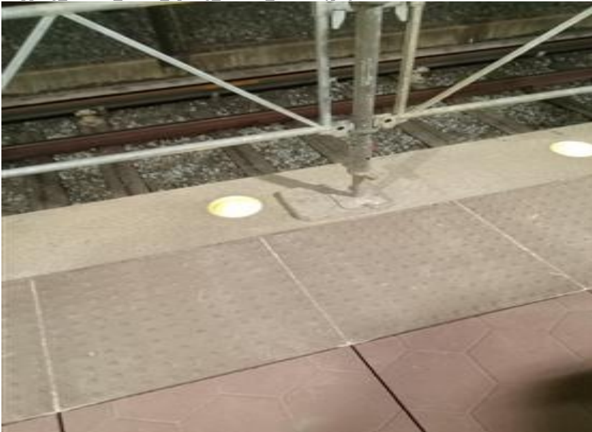
Tripping Hazard Silver Spring Station_082824.jpeg
