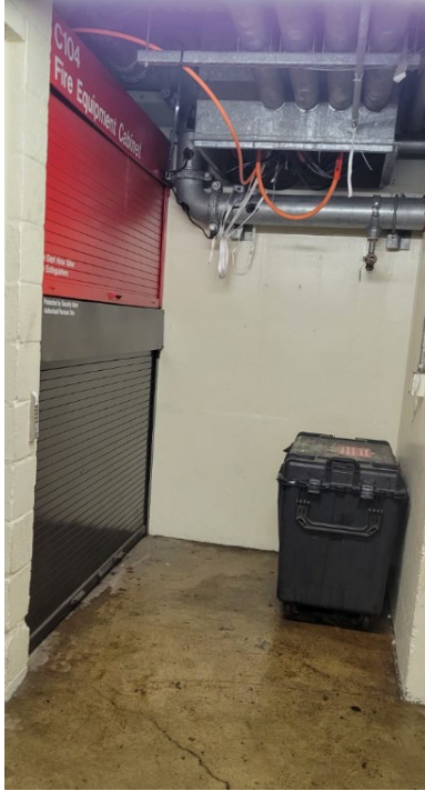
Fort Totten emergency Cabinet C104 corrected by Station Manager
