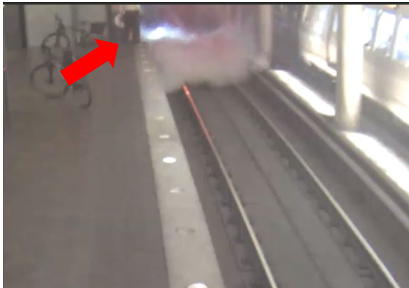
Figure 3 MTPD Personnel attempting to extinguish Arcing Stud Bolt at F03
