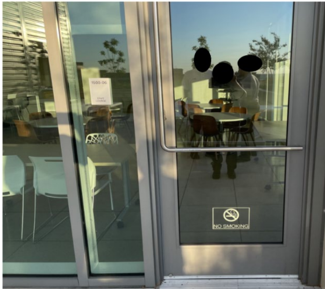
Image 13: Penthouse door displaying a no smoking sign leading to the kitchen (post-fire).
