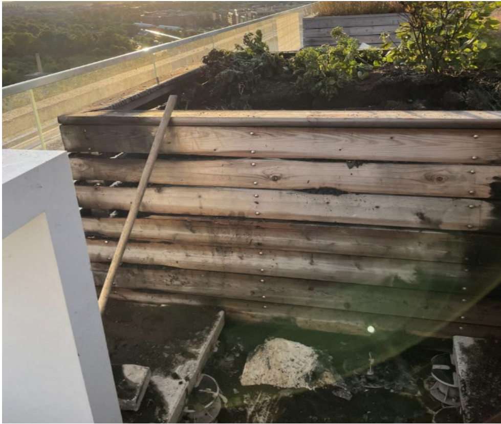
Image 8 – Image of the damaged wooden flower planter.
