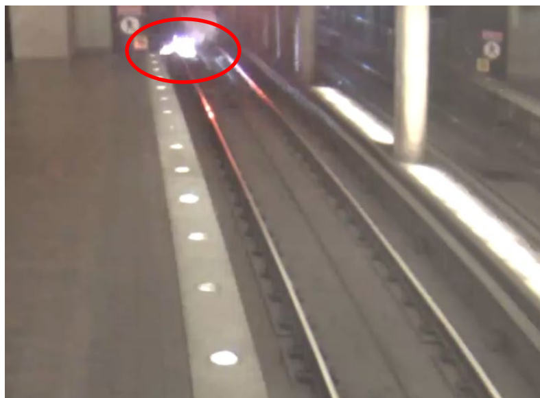
Figure 1 Arcing Stud Bolt at F03 Track 1
