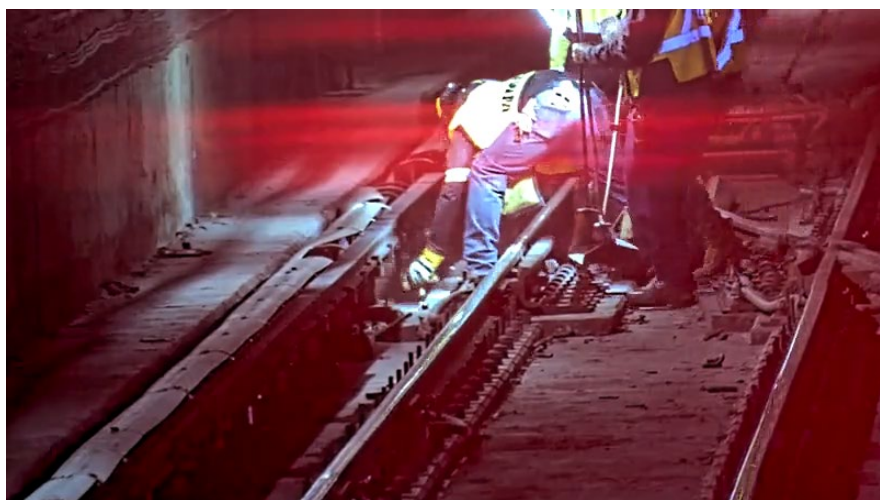
Figure 7 - depicts ERT clearing the debris underneath the third rail from the roadway
