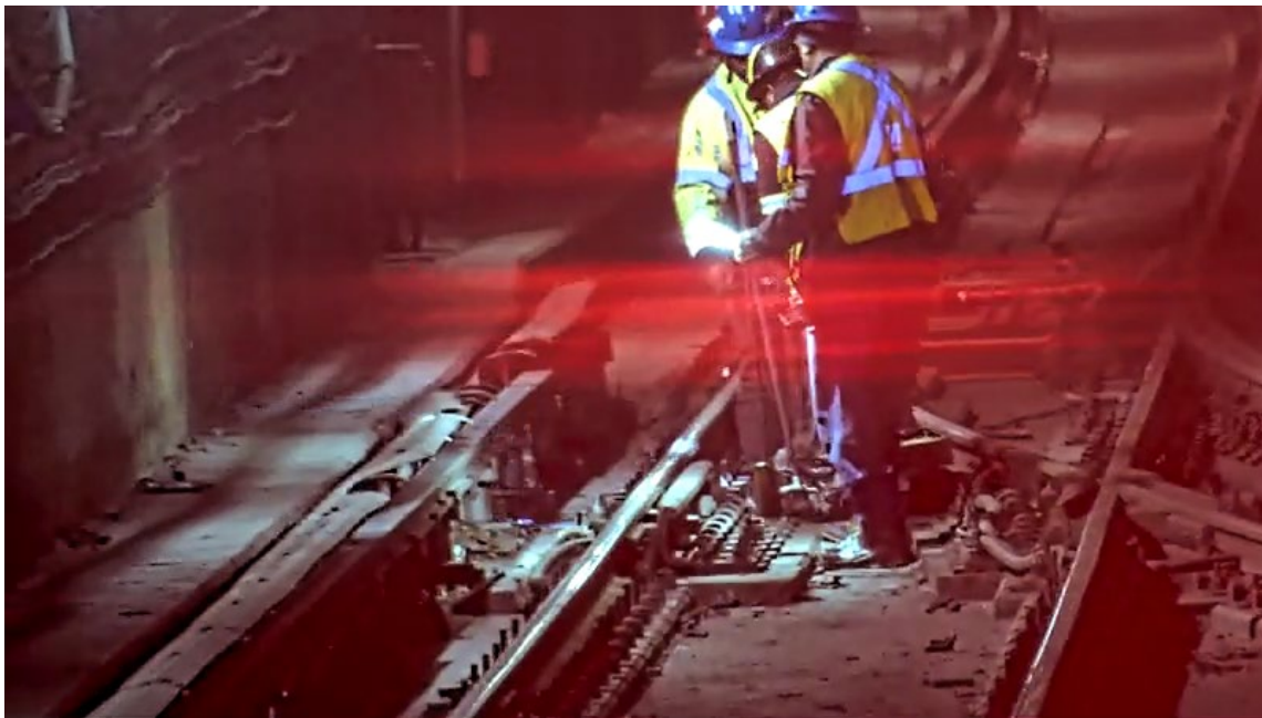
Figure 18 - depicts ERT personnel clearing the debris near the third rail on track 2
