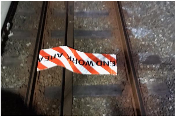
Photo 3: End work area mats installed in joint occupancy without lights.
