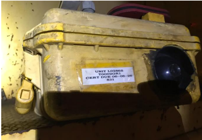
Photo 4: Uninstalled WSAD located on the associated prime mover.
