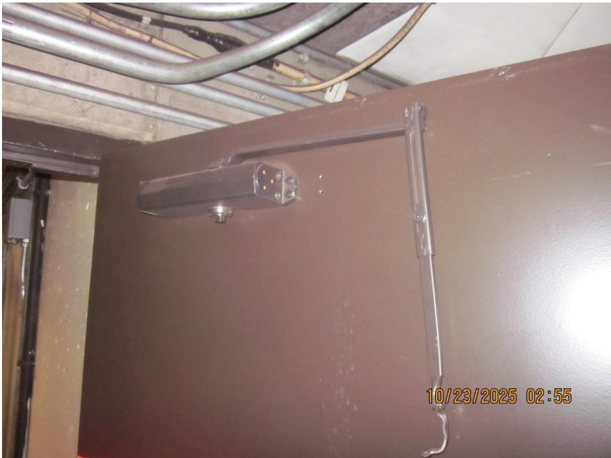
Photo 3: Broken fire door.
