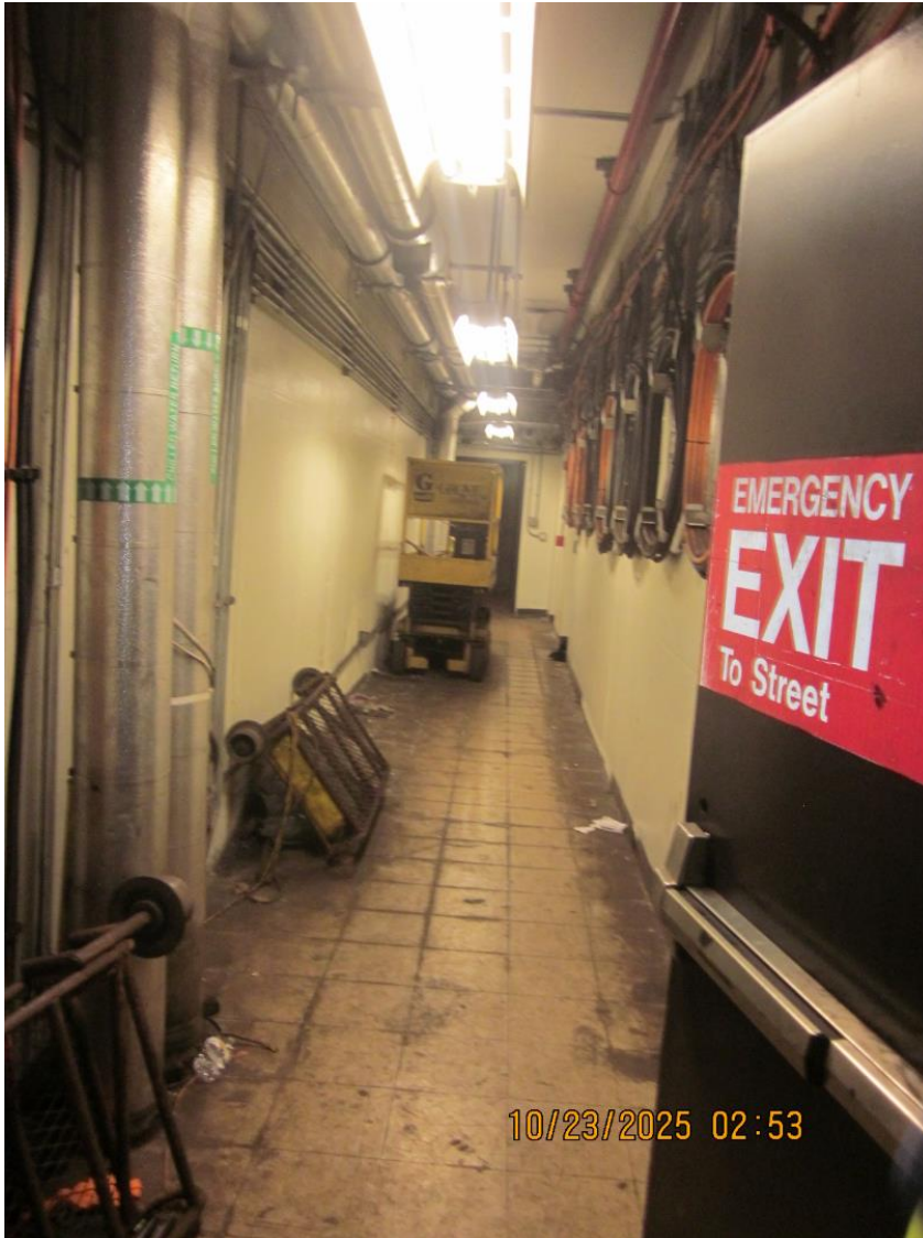
Photo 1: Emergency egress room 104 (hallway) blocked by equipment broken fire exit door.
