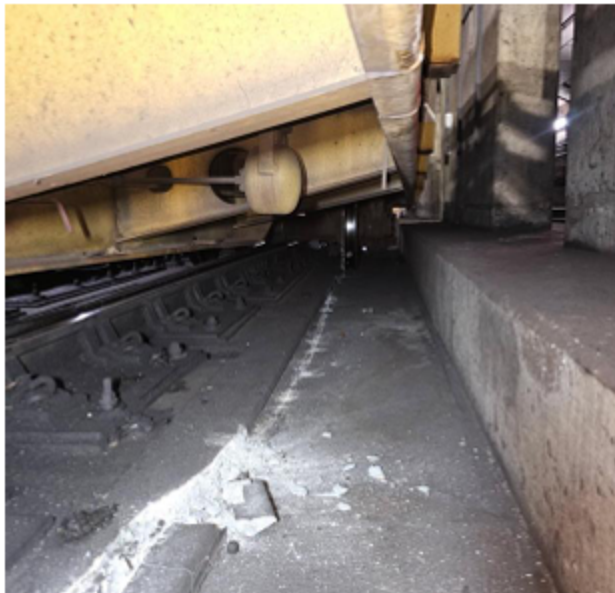
Figure 1. Derailed F606, concrete damage
