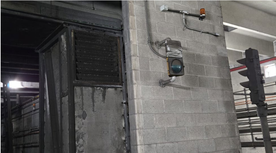
Photo 4: Signal covered by duct tape.
