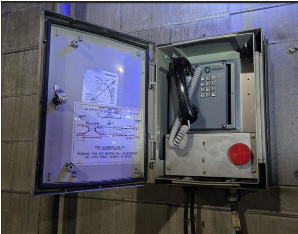
Photo 6: Inoperable phone on ETS box B231.
