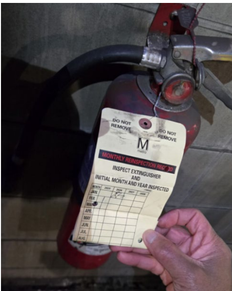
Photo 5: Fire extinguisher that requires inspection.
