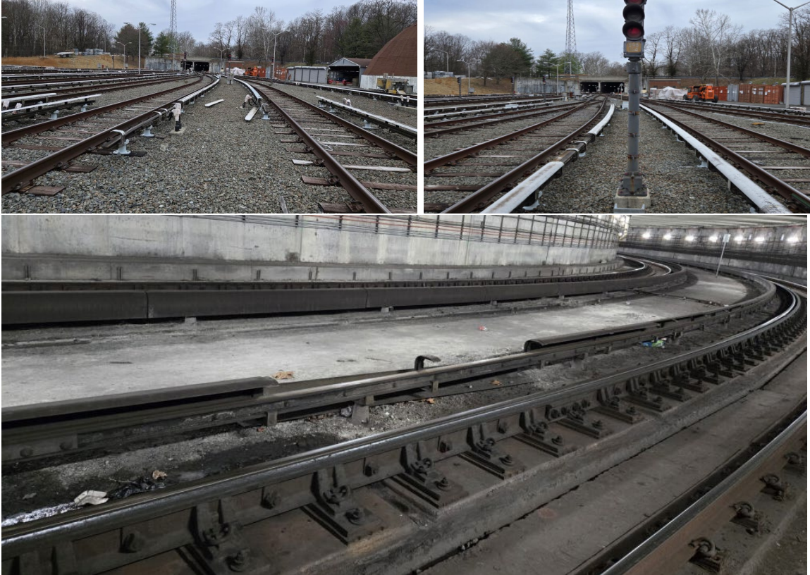
Photos 1 (upper left), 2 (upper right), and 3 (bottom center): missing third rail cover boards.
