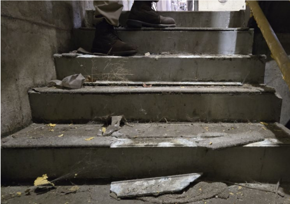
Photo 11: hazardous condition on car wash steps.
