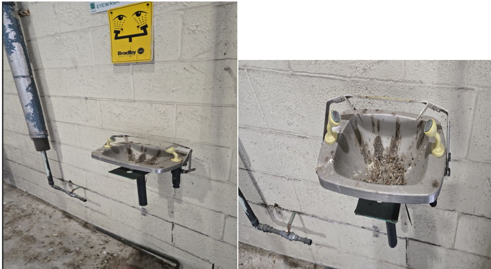
Photos 4 (left) and 5 (right): Disconnected decontamination station filled with debris.
