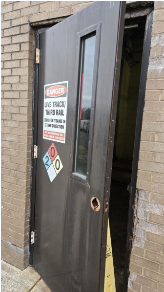
Photo 1: Exterior door without knob or lock mechanism and propped open.
