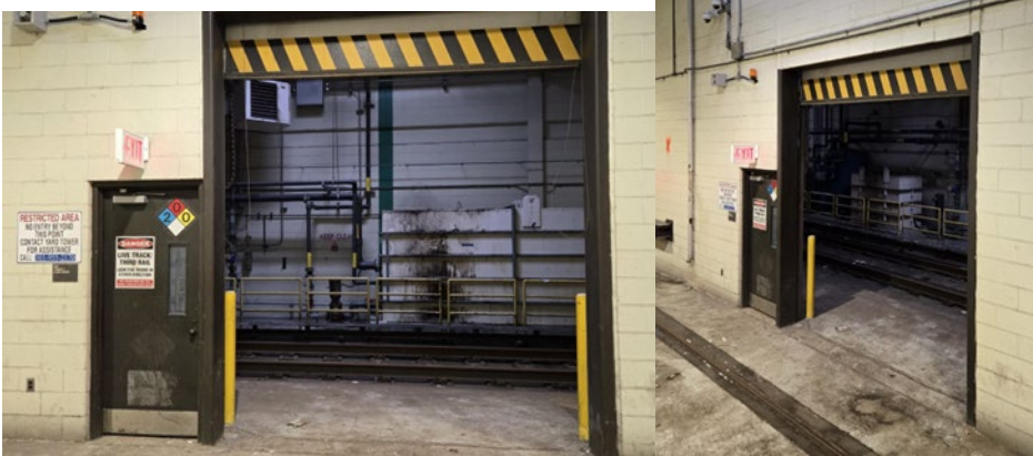
Photos 2 and 3: Unsecured roll-up door between the S&I shop and the car wash facility.
