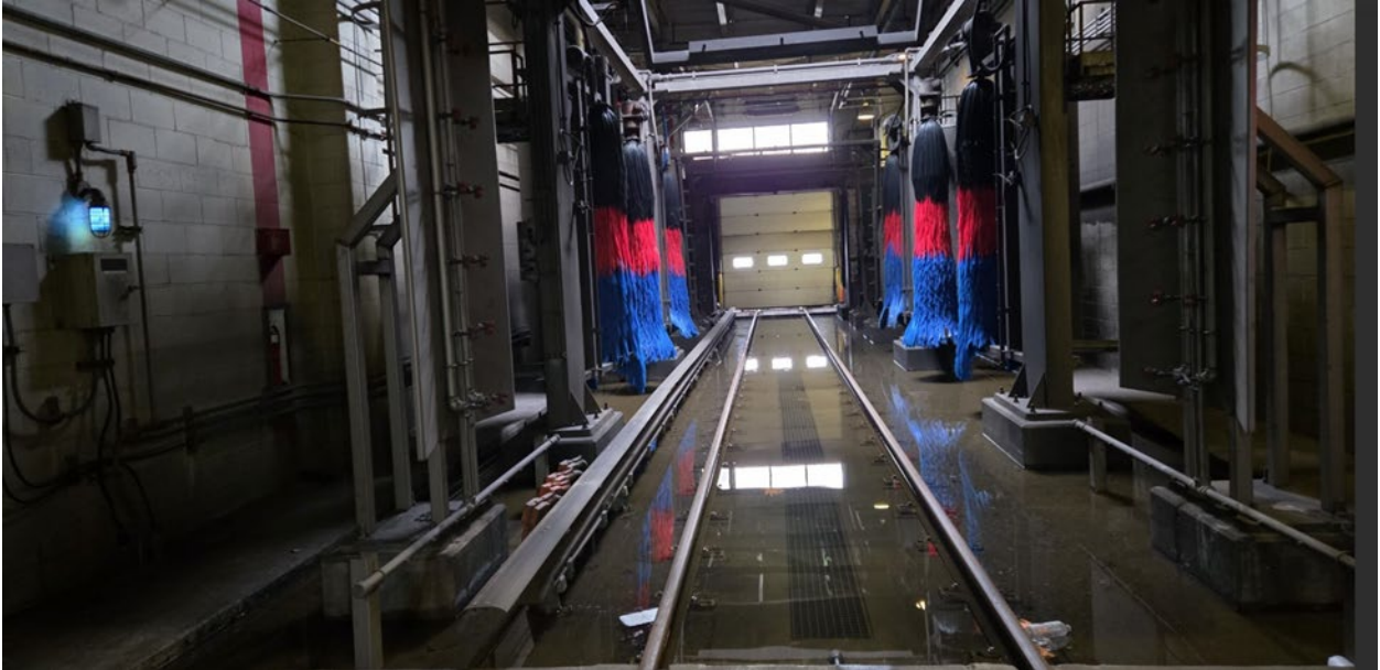
Photo 1: Interior of the Greenbelt Yard (E99) car wash.
