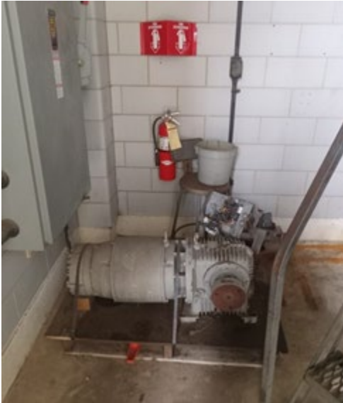
Photo 5: Equipment stored directly in front of the fire extinguisher.
