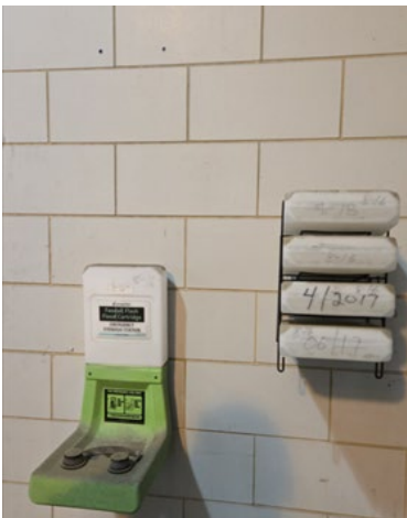
Photo 4: Eye wash station missing signage.
