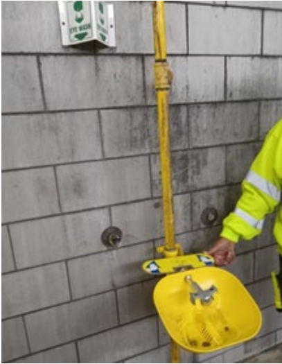
Photo 6: Non-functioning eye wash station.
