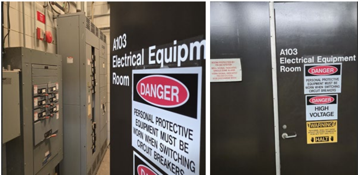
Photos 1 and 2: The unsecured A103 electrical equipment room that has since been fixed.
