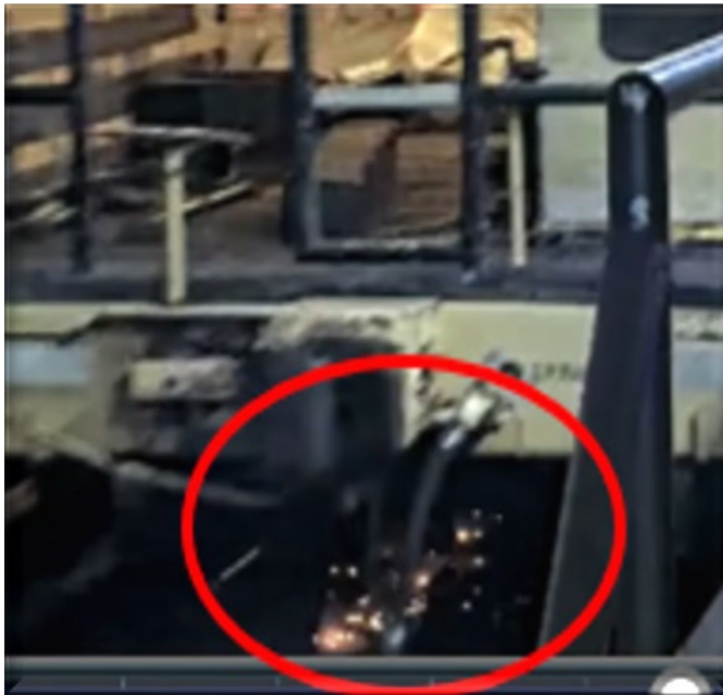
Figure 3 - Image of sparks coming from the undercarriage of Flatcar F606.
