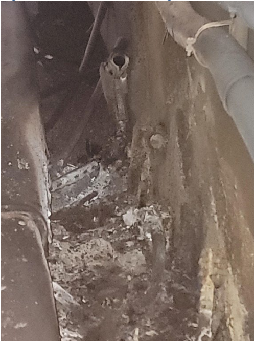
Figure 6 - Residual fire damage to the tunnel wall and roadway.
