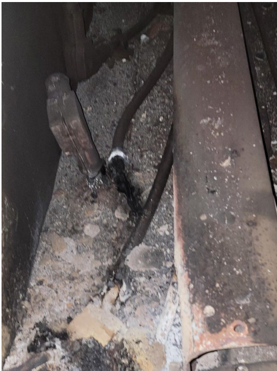
Figure 4 - Black booted pothead cover and electrical wire damage.
