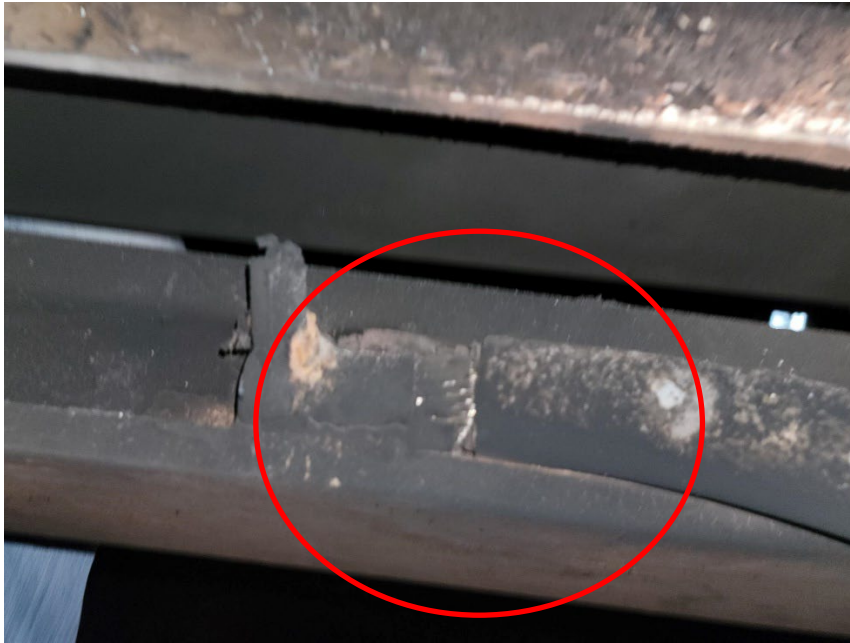
Figure 16 - A close-up of a crack in the metal structure.
