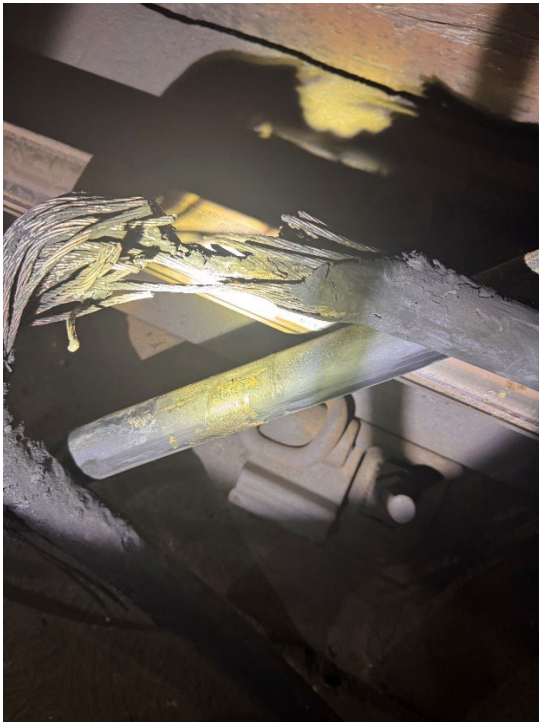
Figure 5 - Electrical wire damage.
