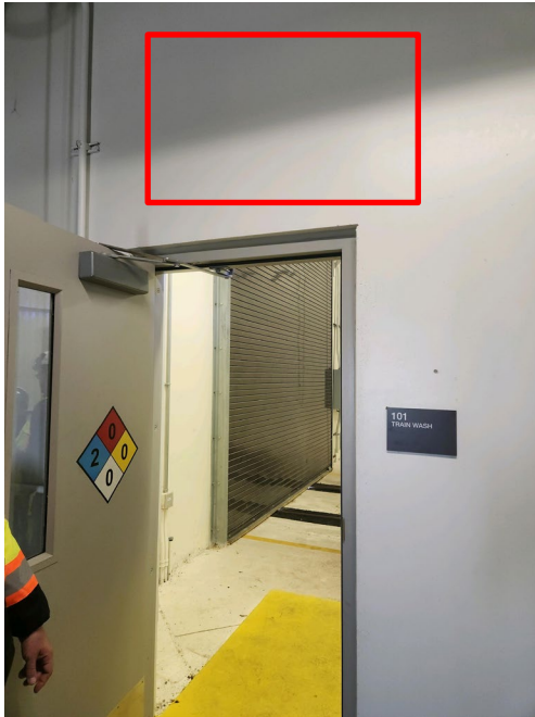
Photo 5: Doorway missing any warning system to alert workers they are entering an area of the building with potential rail vehicle movement.
