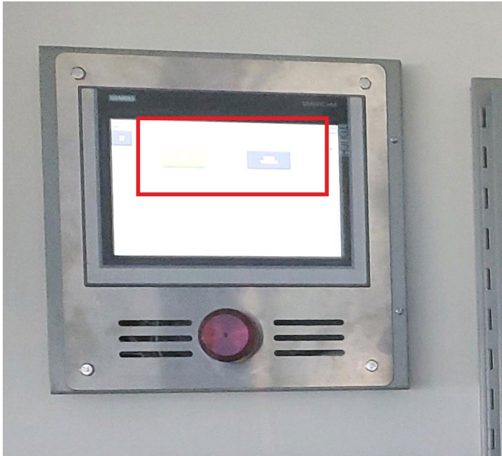
Photo 7: Out of service control panel in the Tower.
