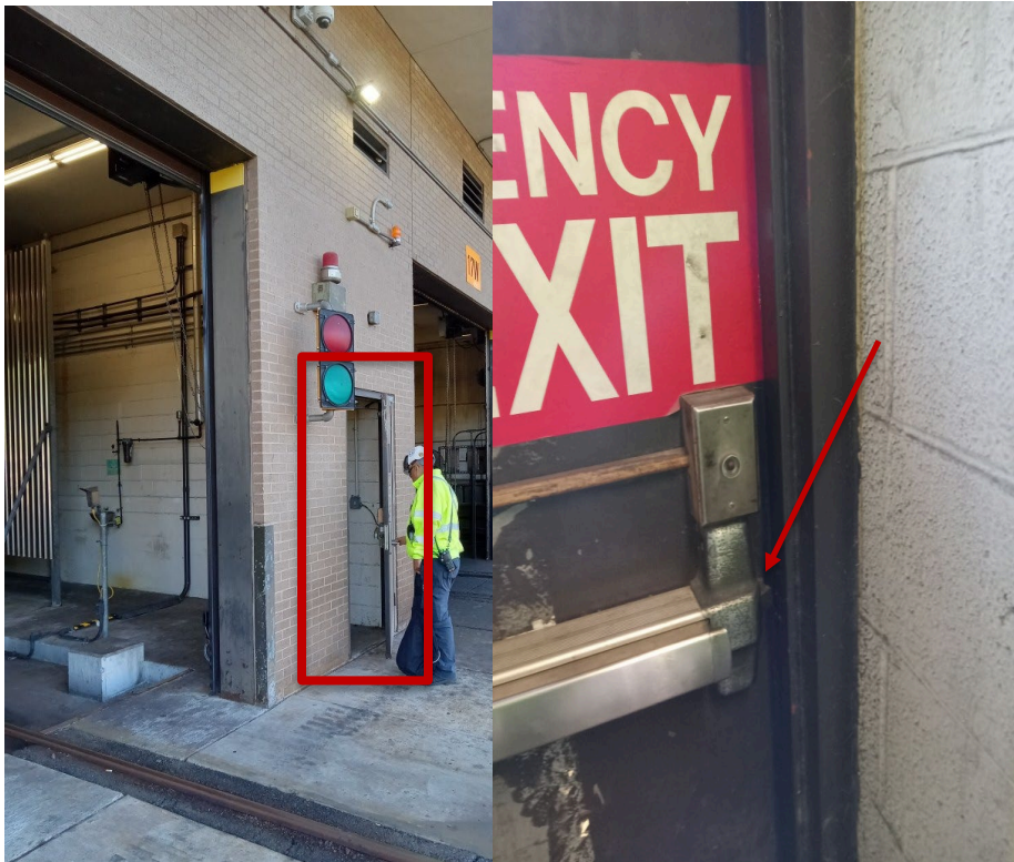
Photos 3 (left) and 4 (right): location of exterior door and the latching mechanism that is not functioning.
