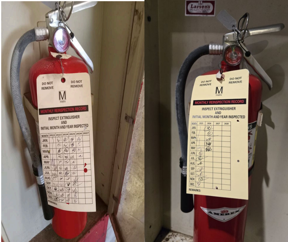
Photos 1 (left) and 2 (right): extinguisher that needs to be inspected for May 2026 and an example of one of the four extinguishers that already completed the May 2026 inspection.
