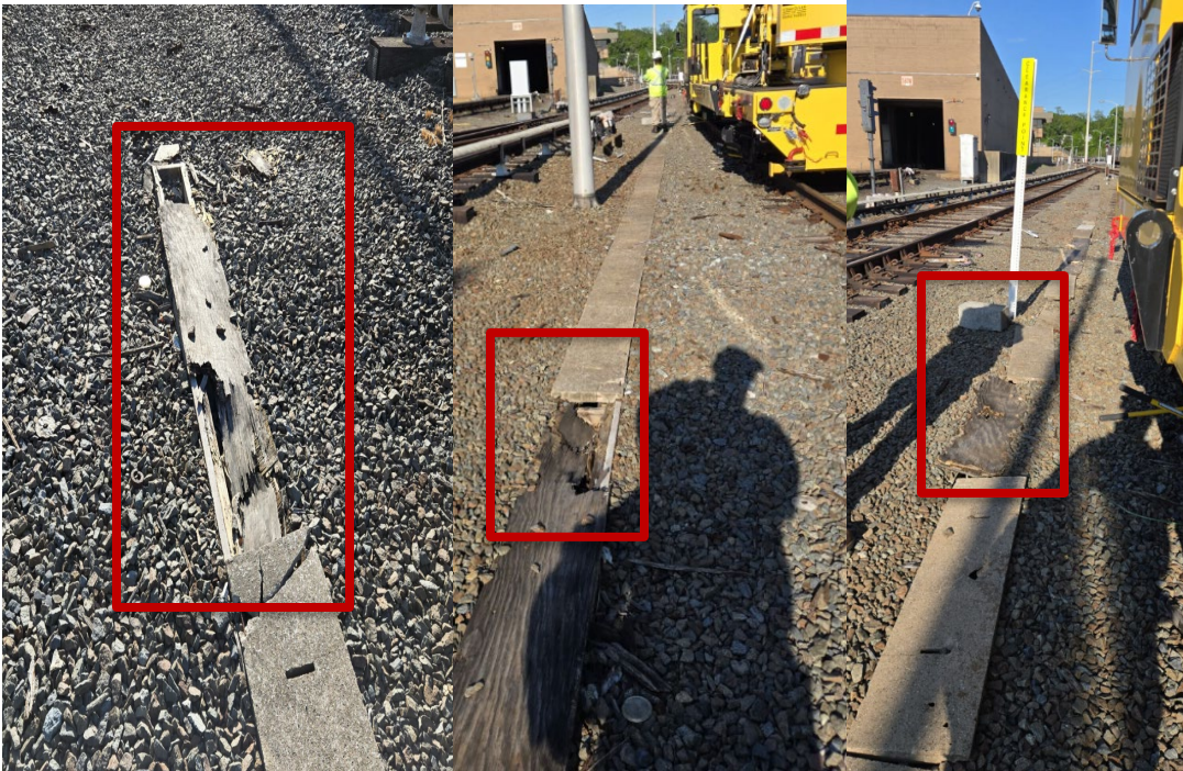
Photos 9 (left), 10 (center), and 11 (right): Photos of the damaged, broken, or deteriorated covers.
