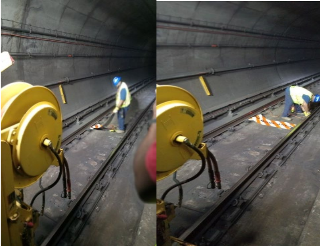
Photo 7 (left) and 8 (right): RWIC properly placing shunts and work zone mats during the work zone set up.
