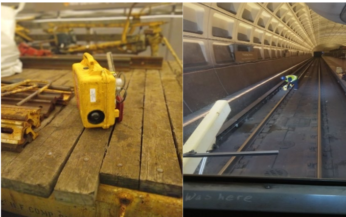
Photo 10 (left) and 11 (right): The Wayside Strobe Alarm Device (WSAD) with a calibration date of 7/29/26 and the RWIC's proper installation of the device.
