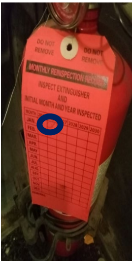
Photo 2: Fire extinguisher with expired inspection tag located in the Flag Person's booth (F607) on the flat connected to PM47
