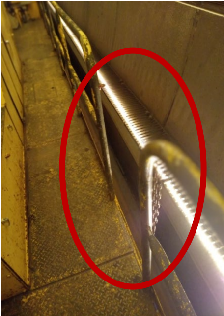
Photo 3: Unsecured Chain Link on PM47.
