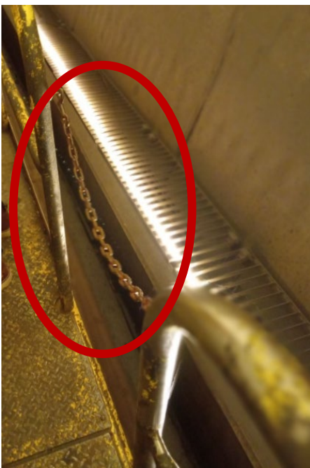
Photo 4: Issue mitigated by onsite staff and the chain link properly connected on PM 47.
