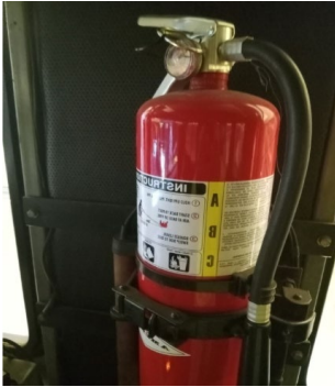
Photo 1: Fire extinguisher with missing inspection tag located in the cab of PM47.
