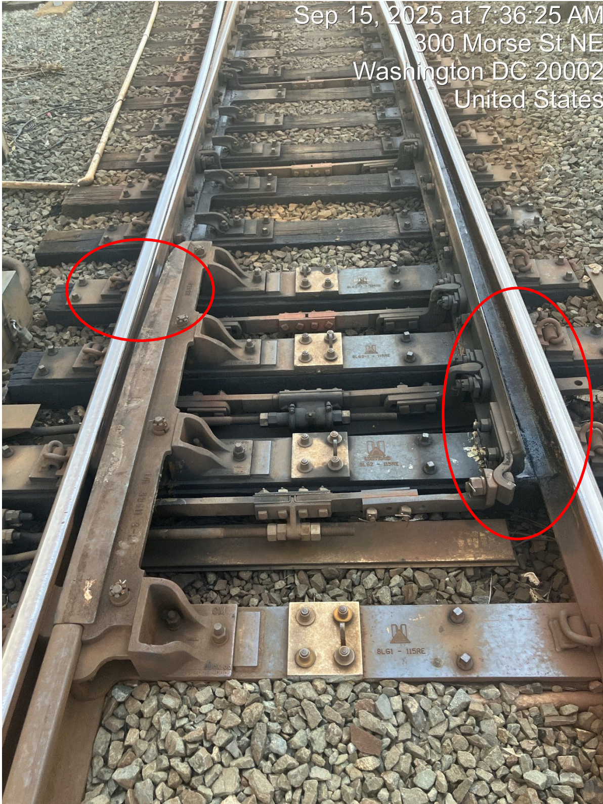
Image 6: Depicts switch 7A point with no damage
