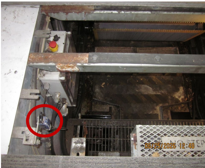
Photo 4: Limit switch in C06X02 pit.
