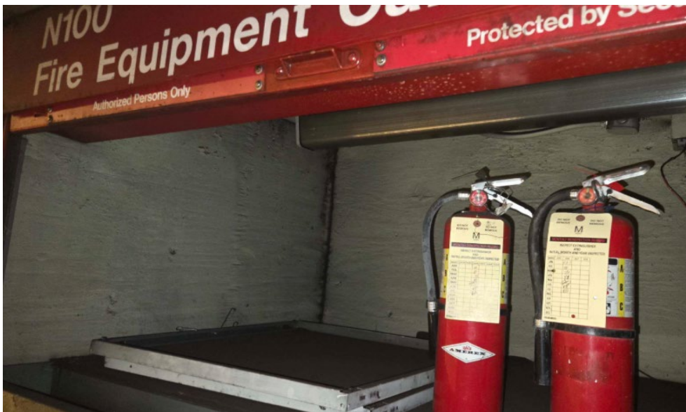
Photo 14. Non-fire equipment items stored in the fire equipment cabinet.
