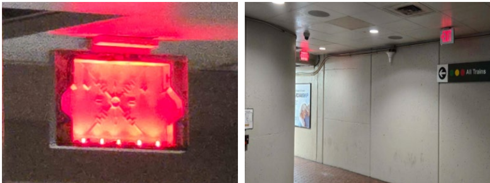
Photos 3 and 4. Exit sign damaged and location.
