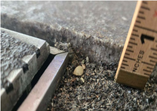
Photo 15. Misalignment at escalator landing.
