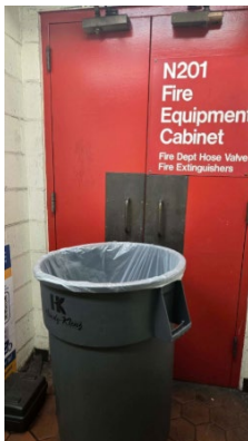
Photo 9. Trash receptacle blocking the fire equipment cabinet.
