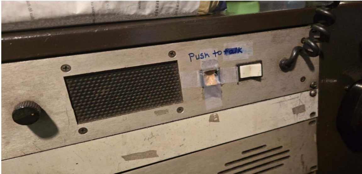
Photo 1. Nonfunctional public address system showing a missing button and covered with tape.
