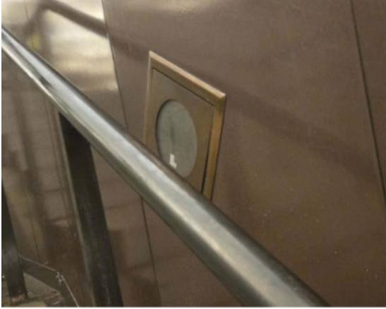
Photo 5. One of many lights observed on escalators that was not illuminated.
