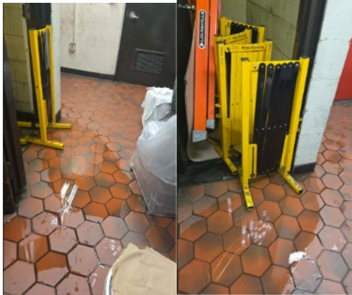
Photos 12 and 13. Presence of water.
