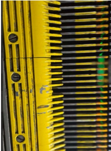
Photo 15. Comb teeth missing on escalator N05.
