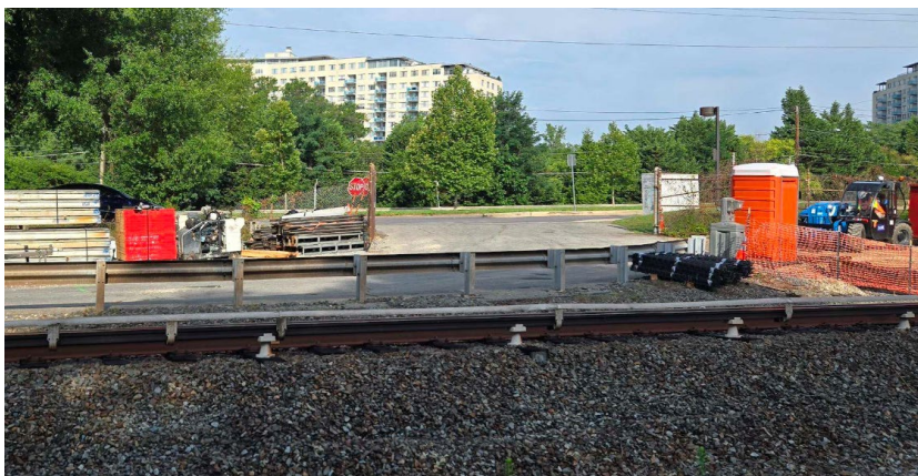
Photo 6: Unsecured and open area to the ACS, easily accessible from Rockville Pike – MD 355.
