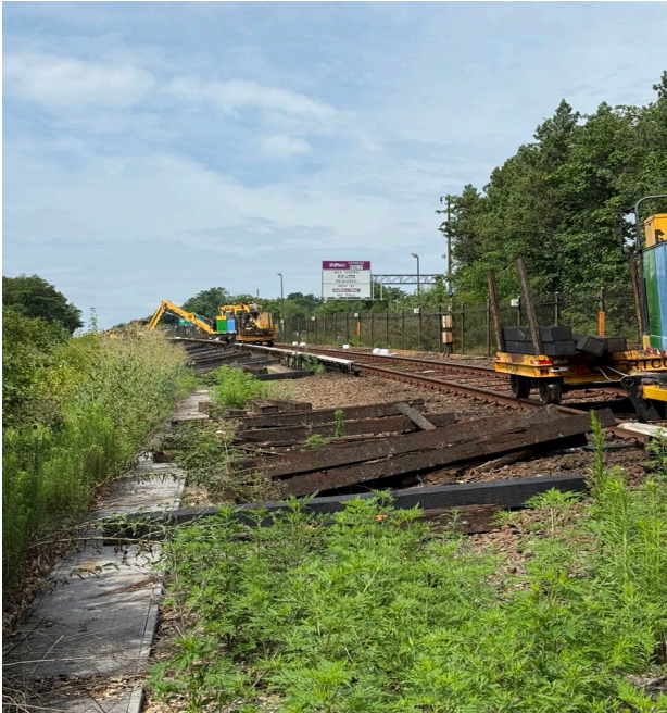
Photo 7: Work site involving multiple tie equipment that would traverse the work site (these are one type of roadway maintenance machine) with no watchperson present.
